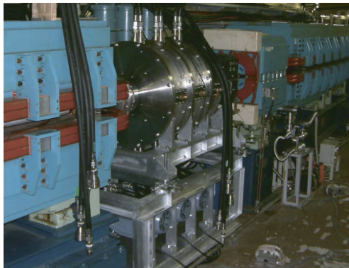
Repetitive induction modulator installed in KEK 12 GeV PS
