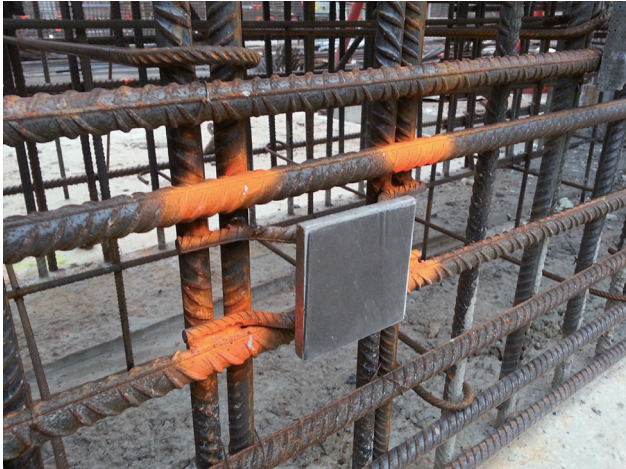
Fig. 41. Iron re-bar earthing mesh within the concrete walls, floor and ceiling of ELI Beamlines experimental facility. A grounding plate is also shown.
