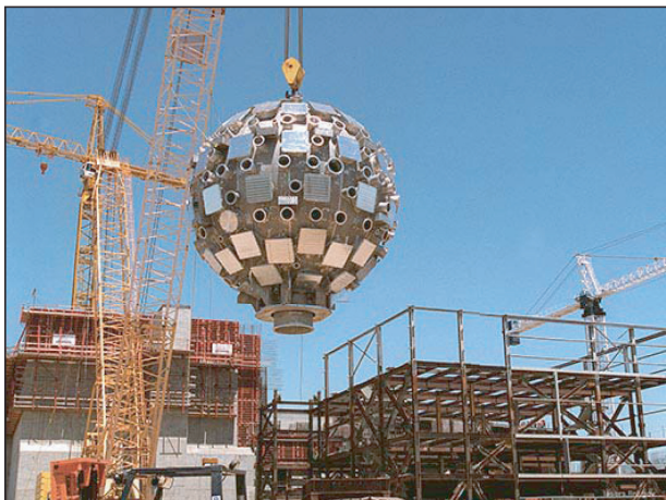
Fig. 9. NIF target chamber prior to installation in the NIF building. The ports for symmetric illumination for direct drive are clearly visible.
