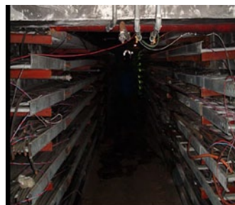
Fig. 2 Photo of the fire simulation experiment cable tunne.
