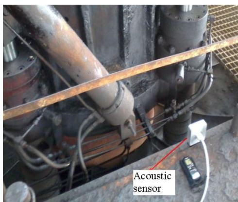
Fig. 3 Acoustic emission sensor of Wuhan petrochemical coke tower experimental installation.
