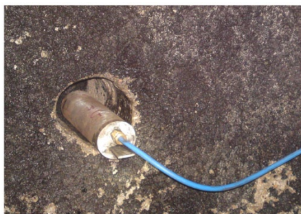
Fig. 5 FBG geophone installed horizontally.
