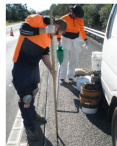
Using a gauge stick to ensure the cable is embedded at the correct depth
