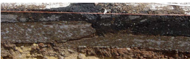
Fig. 3 Example of "stepping" in a road pavement caused by mining induced compressive strain.
