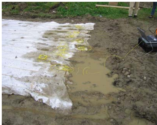
Fig. 13 Sensor-based geotextile mat being installed during construction of a gravity dam in Solina/Poland (textile: Saxon Textile Research Institute (STFI) e.V. Chemnitz).
