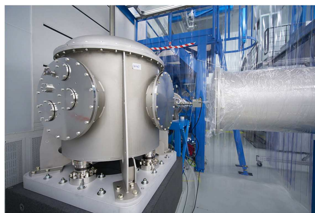
Figure 22. Clean installation in experimental hall E3. Local cleanroom tents were constructed and built to allow clean access to the mirror chambers and to connect them via bellows to the adjacent DN500 pipes.
