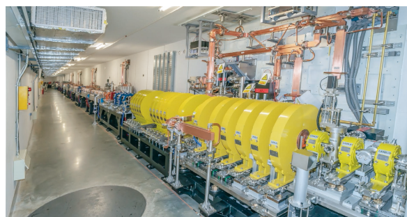
Fig. 1 High Energy Photon Source Linac
