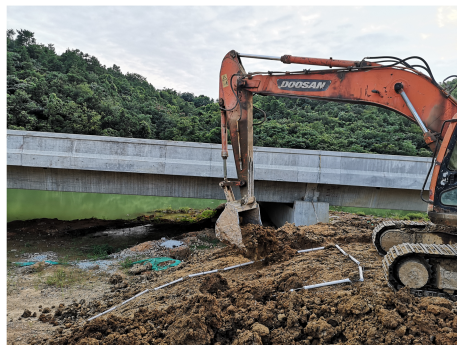
(b) Excavator buries OFSSs in the shallow surface of an artificial slope
