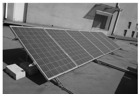
图 1 测试中的屋顶模组(左侧第二片为研究对象) Fig. 1 Solar module under testing on the roof(second module from left side is the object under testing)
