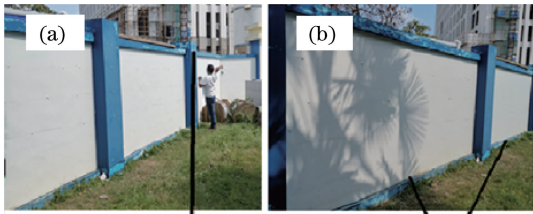
knock on the edge of the wall vibration fiber optic cable
